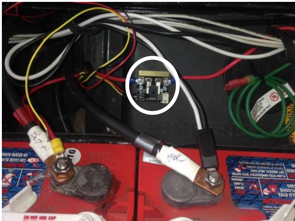
Figure 8. Photograph of where current sensor, circled, is mounted.
